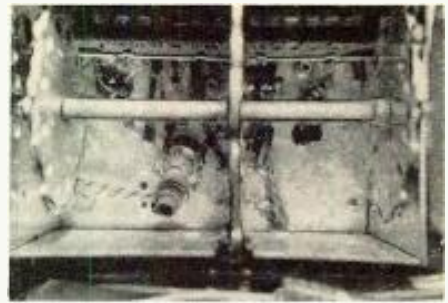
Fig. 4. All strips removed except one pair in use, for access to circuitry.
